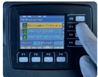
Basic maintenance screen on the 3.5" multi-colour monitor
